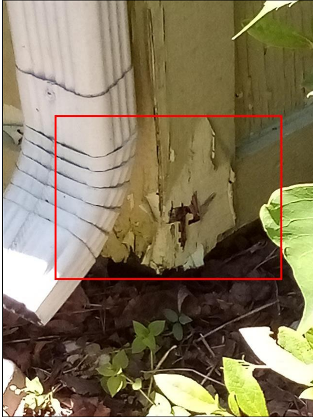
Item 2 - Item 1(Picture) Left rear
